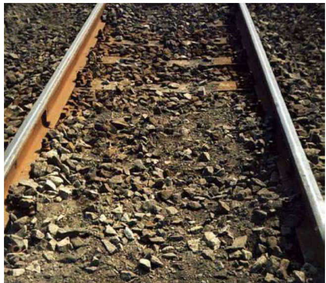
Figure 5. Unacceptable condition of the ballast
