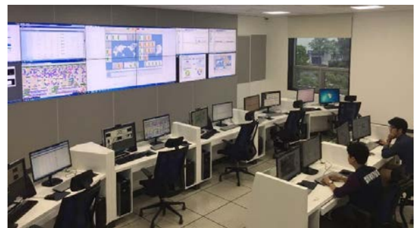
Figure 17. Equipment Monitoring Center in Hyundai motor.
